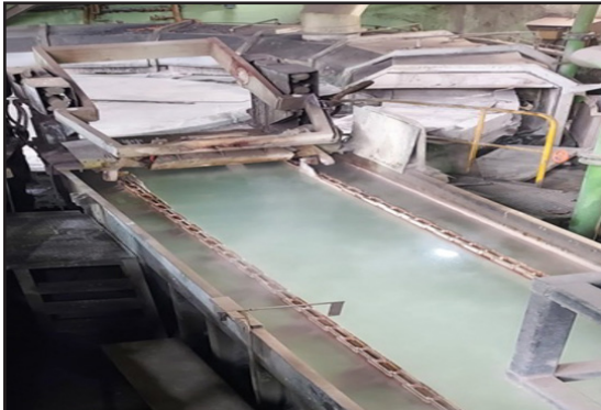
Conveyor chain in copper anode casting pool that is exposed to water and harsh chemicals.
